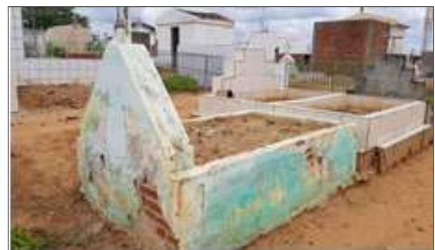
Fig 2: Presence of cracks and fissure – Afogados da Ingazeira – PE - Brazil. Source: The authors.
